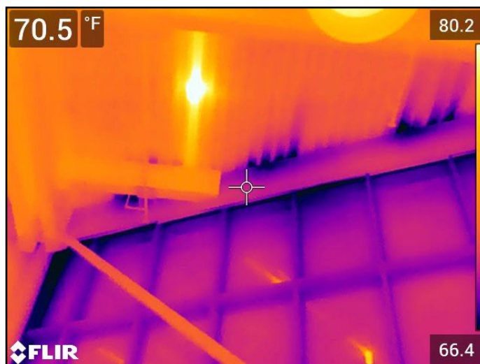
The above image displays cool exterior air leaking to the building's warm interior from pan deck roofing at curtain wall detail. This color array displays presence of an air leak.
