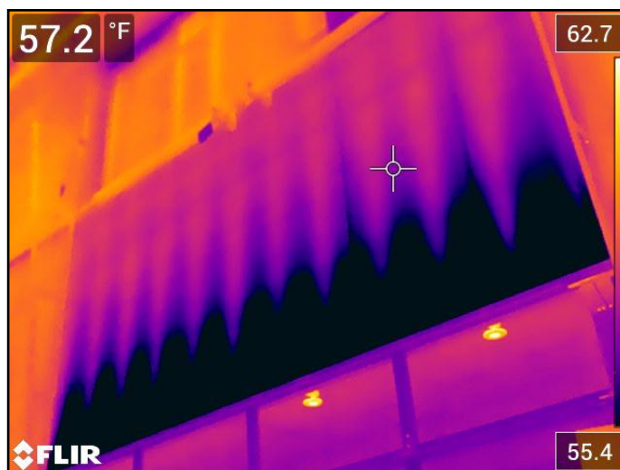
The below image displays cool exterior air leaking into the warm school gym at the head of an overhead door.
